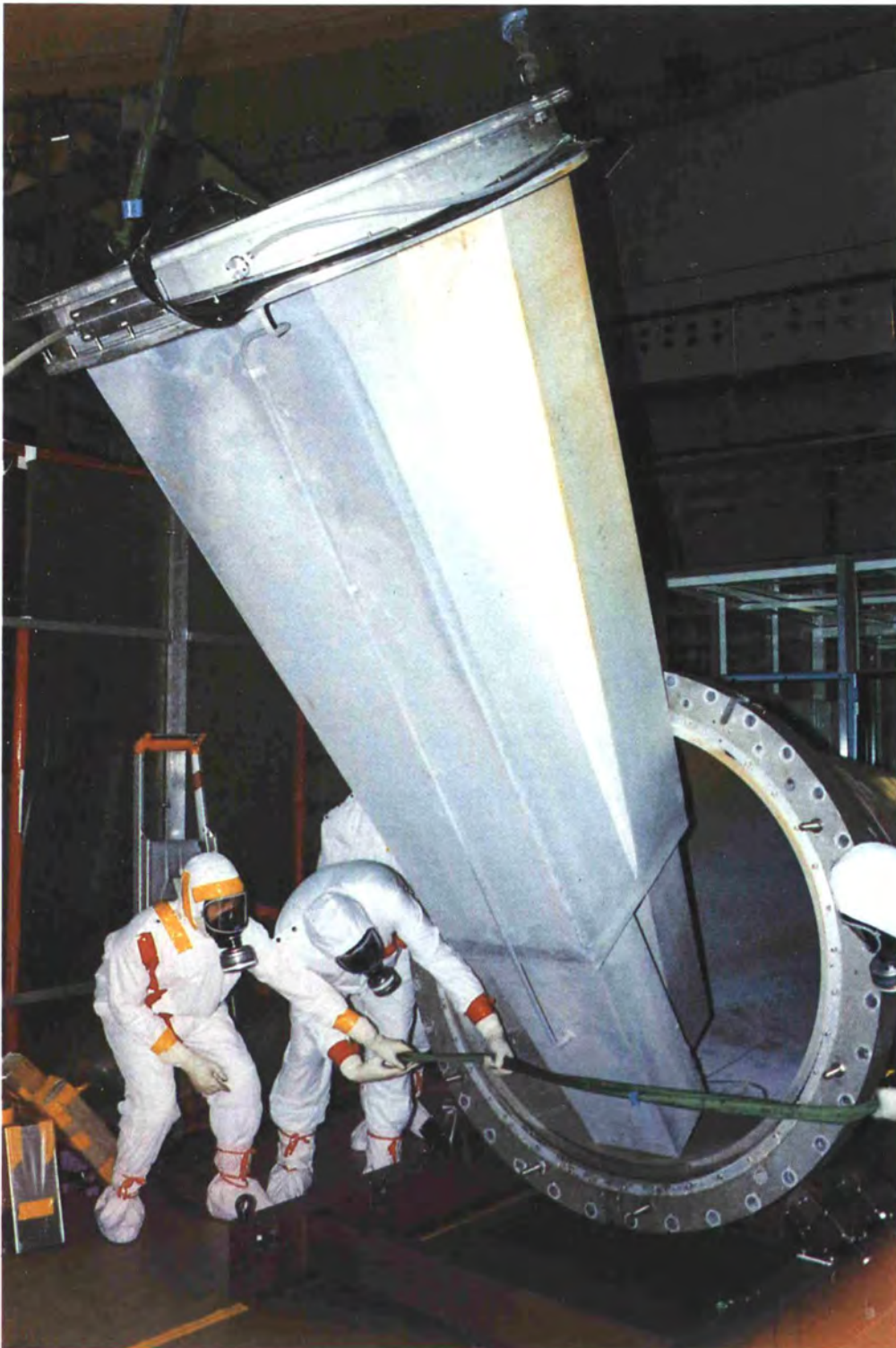
The radioprotection team cleaning the radioactive part of the removed liquid shutter unit of H1/H2.
