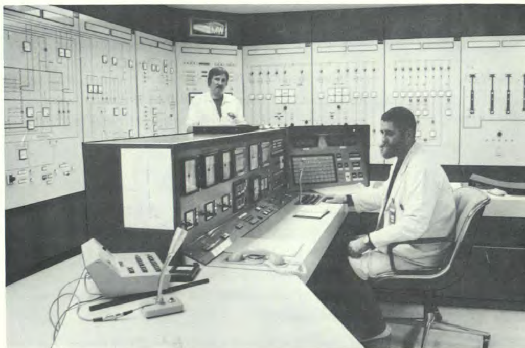
Reactor : Control Room.
