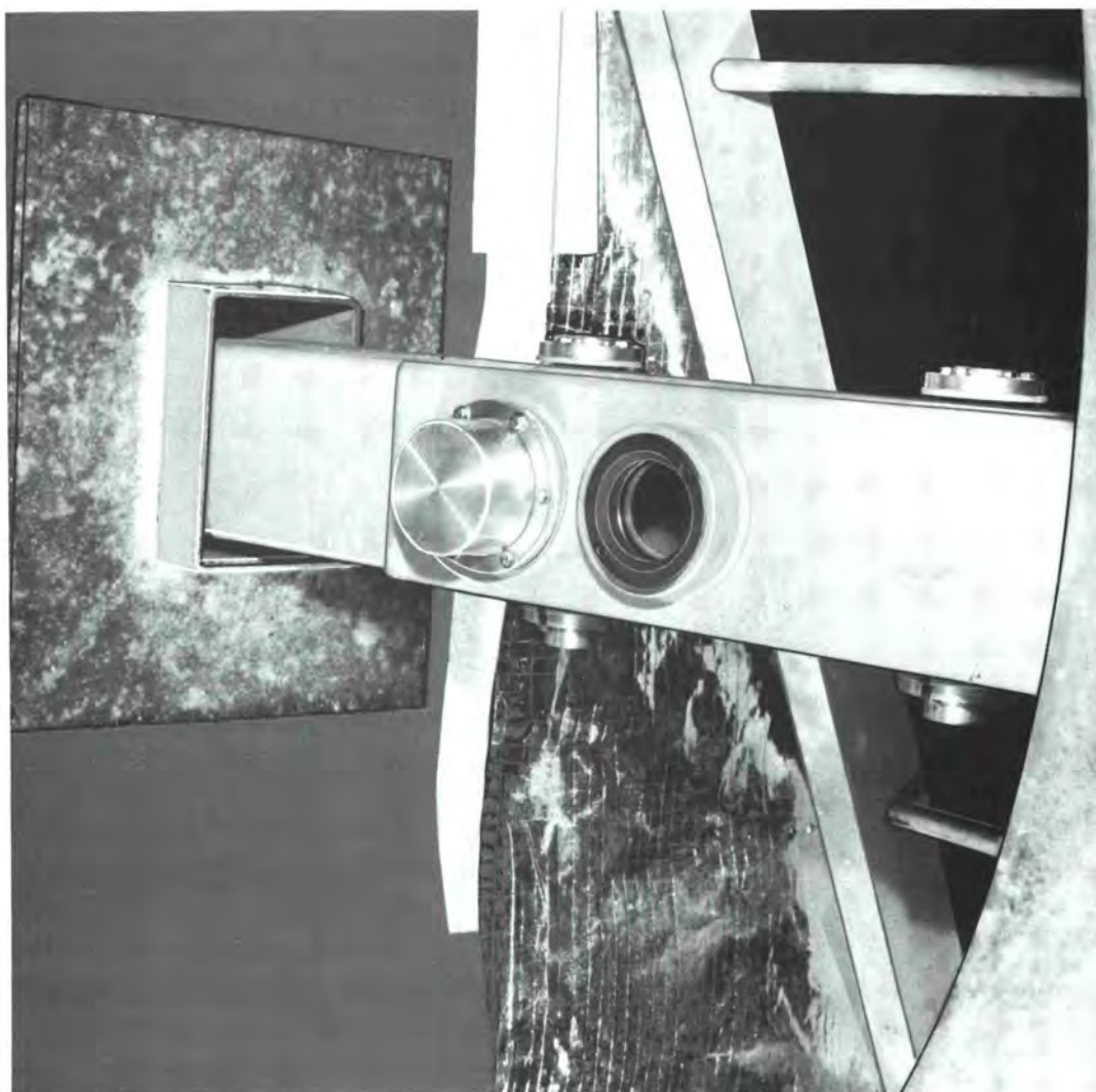
Part of neutron guide for D17, the new small angle scattering apparatus (under construction). The picture also shows the space between the outer (concrete) and inner (steel) shells of the reactor building.
