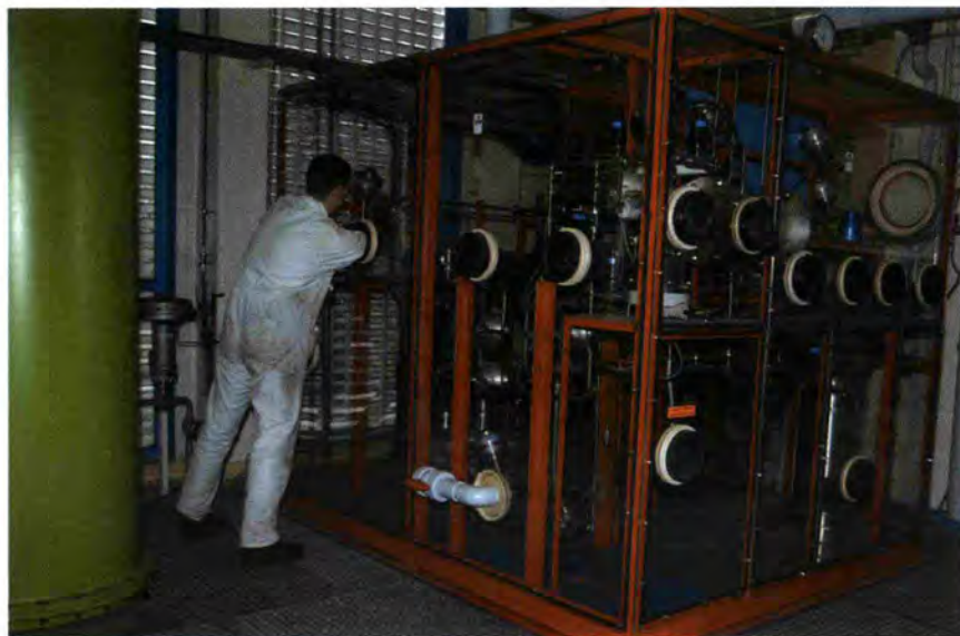
Olivier Aguetaz, technician in the detritiation and source group, at the detritiation station.
