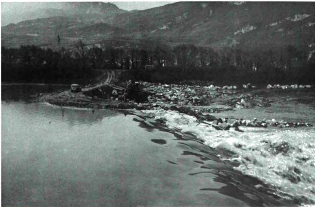
The rockfill dam on the river Drac from which cooling water is drawn for the Reactor. In the background is the temporary dyke built to protect the area where the repair work is in progress.
