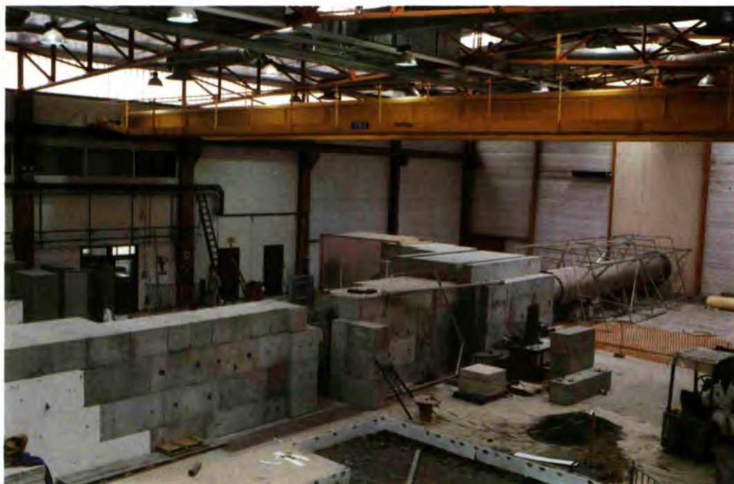
The second guide hall is being fitted out. In the picture (status October 1988) one can see the guide N° H53 feeding IN10C and the n\bar{n} experiment. In the foreground is the foundation for the IN15 tanzboden.
