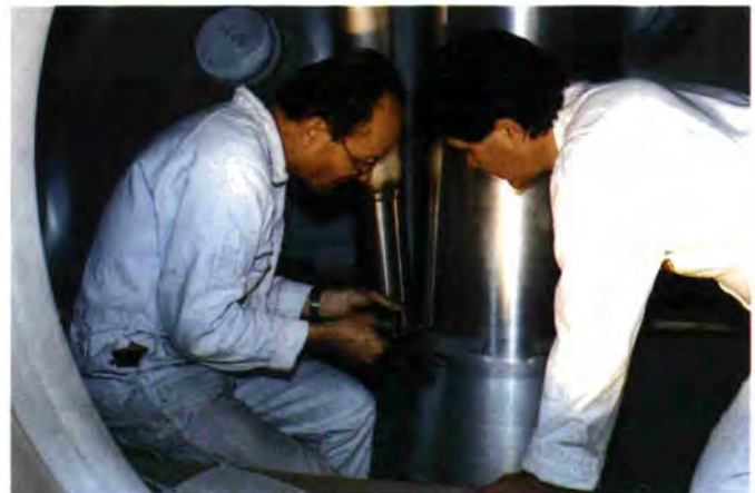
Fig. 21: F. Saint Suplice and A. Rimet verifying dimensions inside the new reactor vessel.
