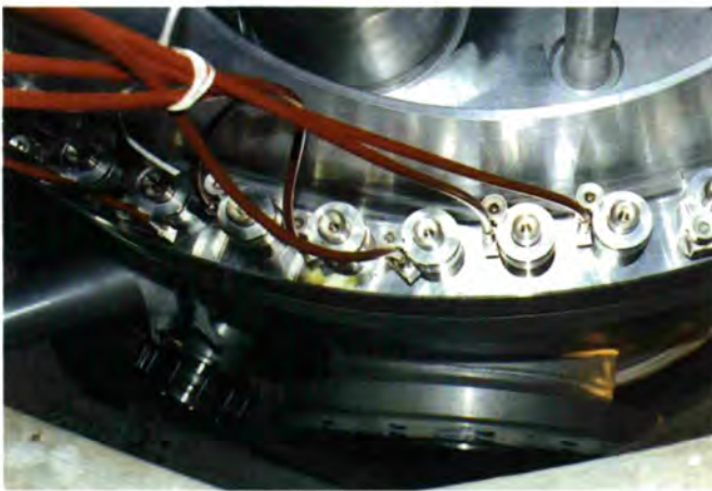
Fig. 19: Hydraulic tightening devices used to close the top of the new reactor vessel.
