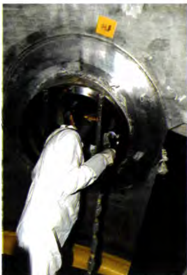
Fig. 16: P. Massafra welding the inner part of a new stainless steel bellows from the swimming pool side.
