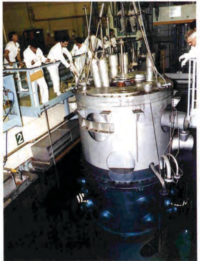
Fig. 1: Transfer of the old reactor vessel to the storage pool with assistance of G. Bonnet, A. Rimet, E. Mannino, J. Correard, M. Selva, J. Fayard, M. Mollier.
