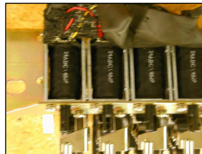
Wiring under insulation behind magnet
