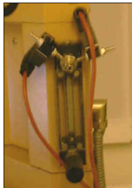
Gas valves fitted to rotameter
