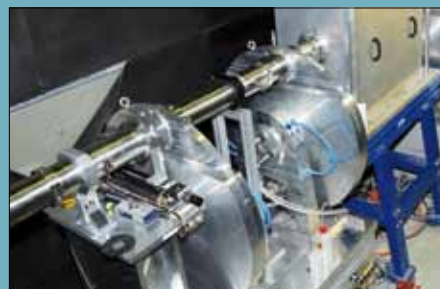
Figure 1: View of the optical casemate for D33 , with its 4-chopper system, velocity selector, and polarising options, inside the stainless steel bunker (roof not yet in position).
