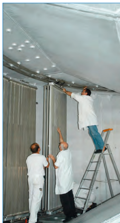
Figure 7: Installation of the detector cassettes inside the flight chamber of the IN5 secondary spectrometer.
